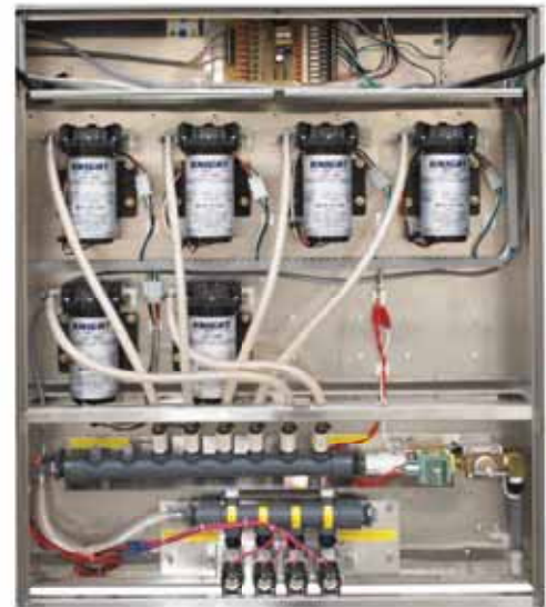
Chem-trak Jr. EDP pump cabinet
